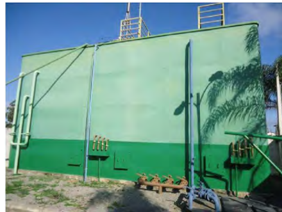
(b) Reator UASB ETE de Solar Bitti
